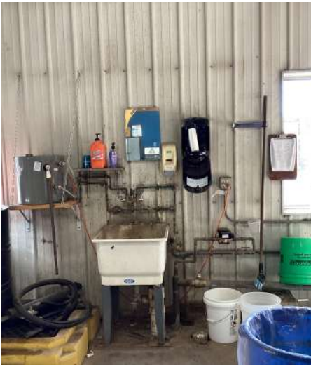
Receptacles/Shop Sink Area
