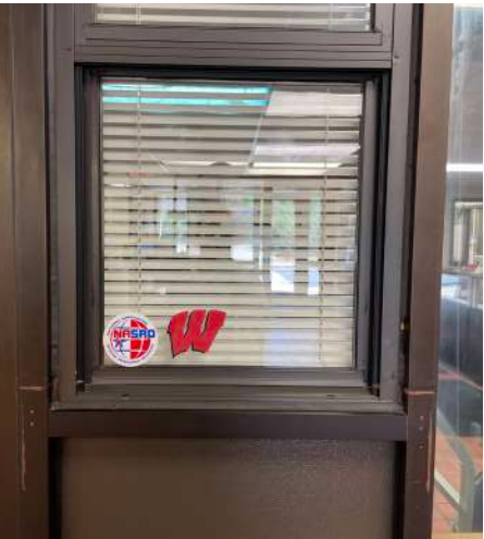
Interior Storefront System
