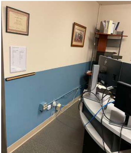
Wall Conduit Court Clerk Office
