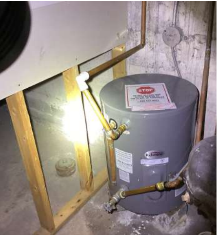
Water Heater/Basement Mechanical Room
