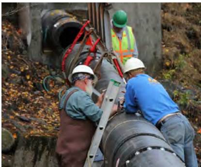
Tighe & Bond's wastewater projects range from small industrial pretreatment systems to large municipal collection and treatment facilities.
