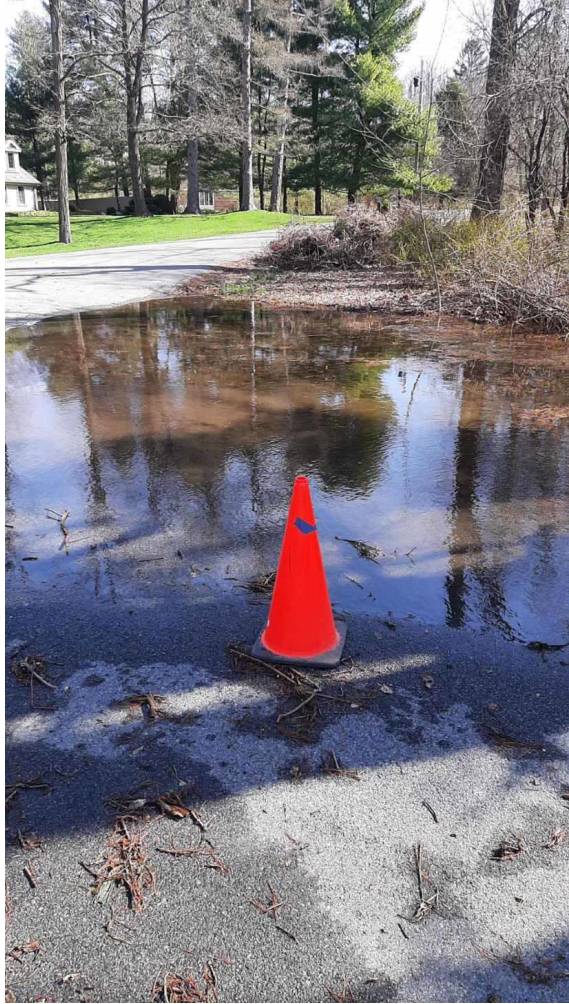
Catch Basin Linden Lane
