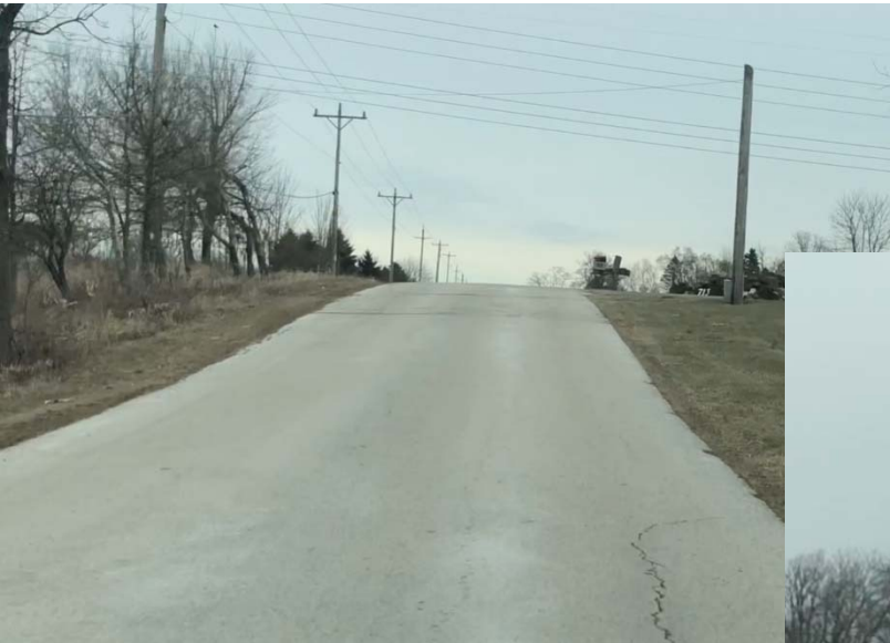
Substandard Vertical Curve Looking West
