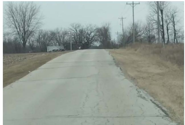
Typical Pavement Deterioration
