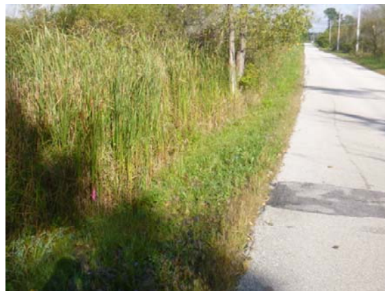
Typical Substandard Shoulder
