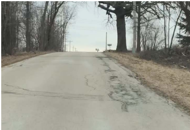
Alligator Cracking and Patching
