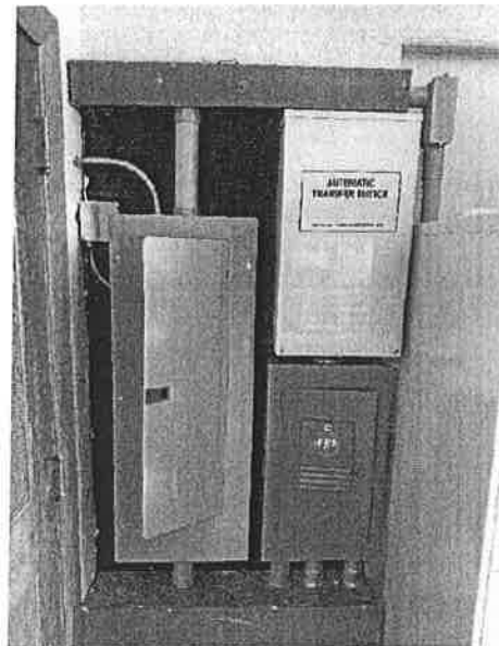
Photo 4 – 1 st Floor Main Electric Distribution Equipment
