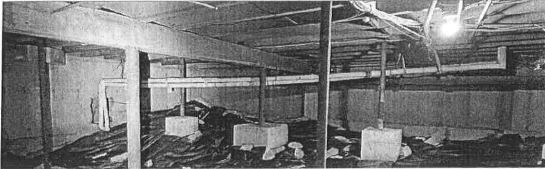
Photo 6 - Well water piping in basement
