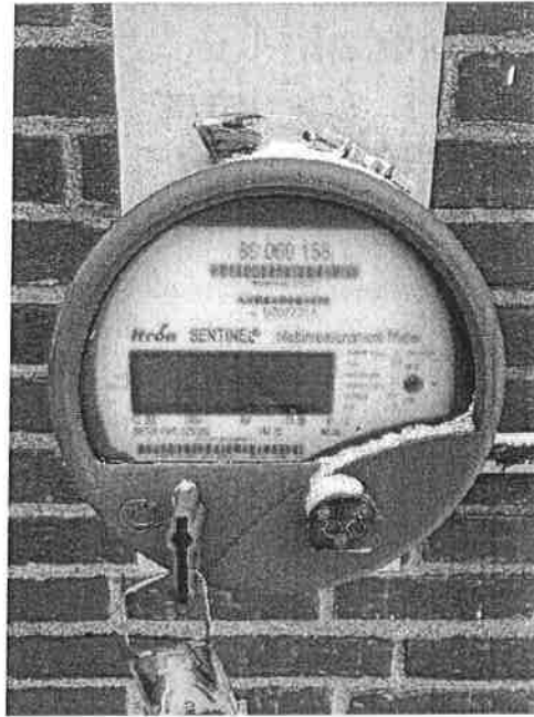
Photo 3 – Utility KW Demand Meter
