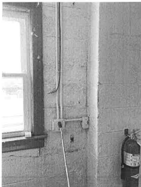
Efflorescence on interior wall of community room
