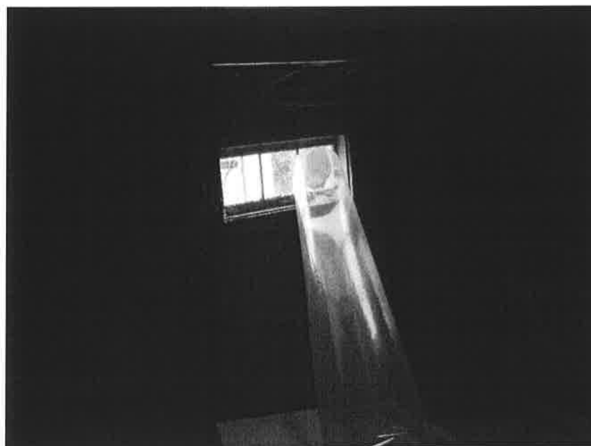
Plastic tube used to vent exhaust air from dehumidifier connected to cellar window
