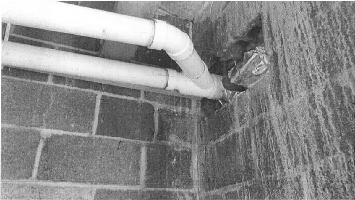
Joined PVC pipes that are combustion air and combustion exhaust vent
