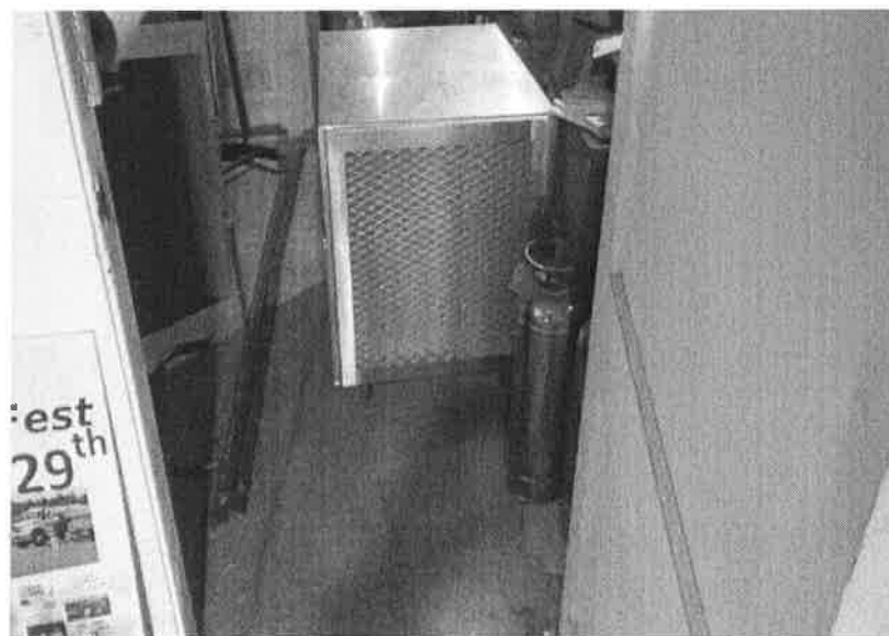
Dehumidification unit in cellar
