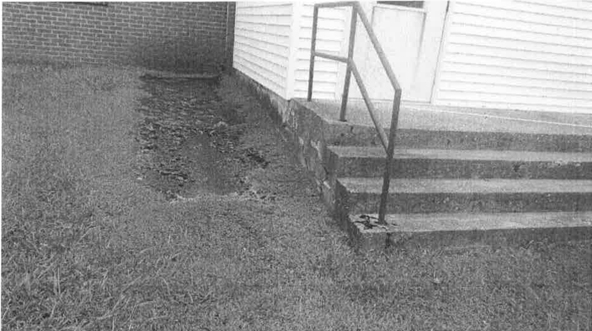
Water accumulation on exterior of front of PTH indicated by dark staining, moss growth, and erosion to brick and mortar
