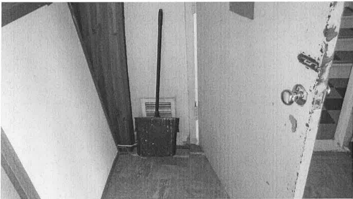
Return air vent
