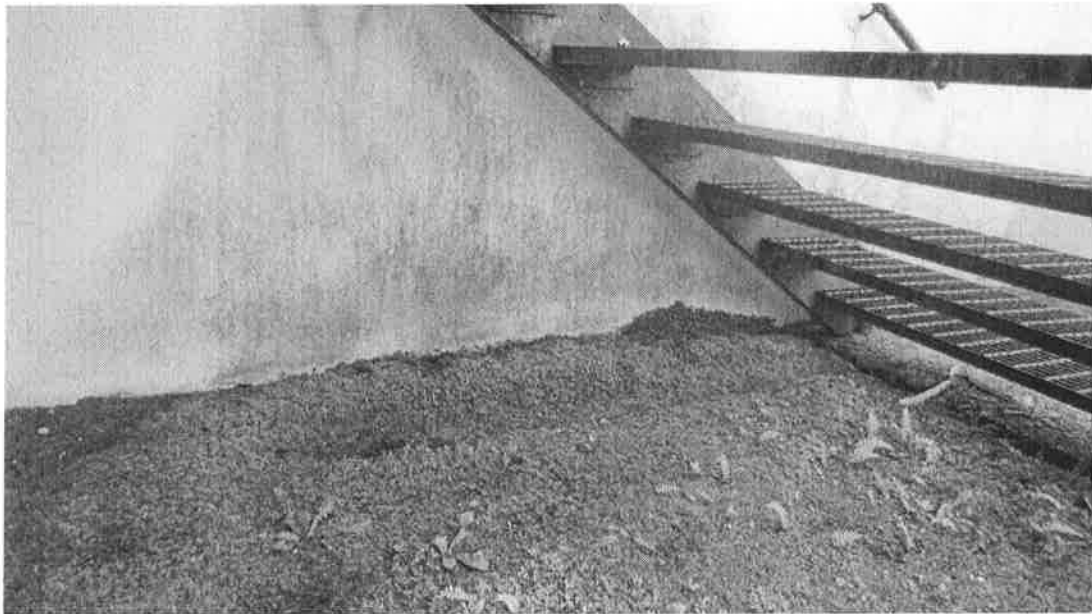
Water accumulation on exterior of rear of PTH indicated by dark staining and moss growth.
