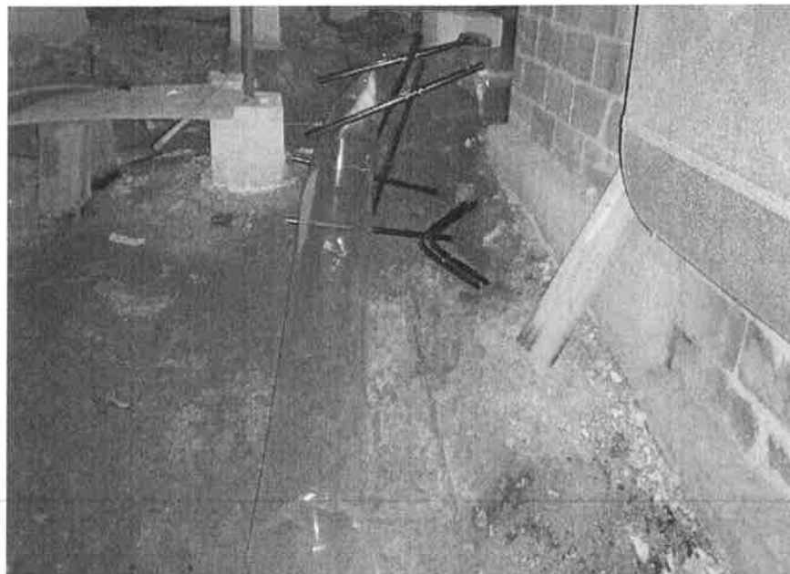
Plastic tube used to vent exhaust air from dehumidifier
