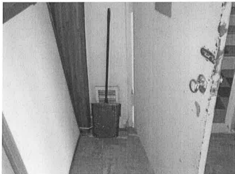
Vent opening in meeting hall
