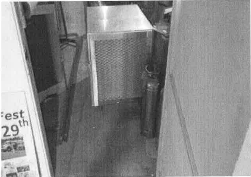
Dehumidification unit in cellar
