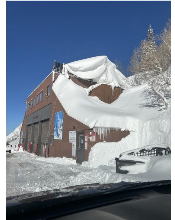
Roofs not rated to support snow load
