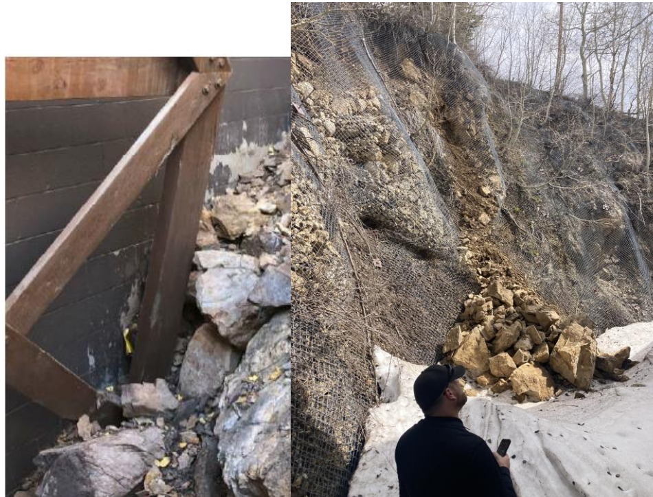
Erosion control efforts have failed. Rockfall is major safety concern and causing building damage.
