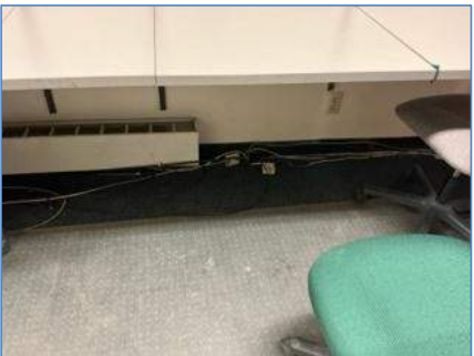
Exhibit 16 – Exposed cables below desks.
