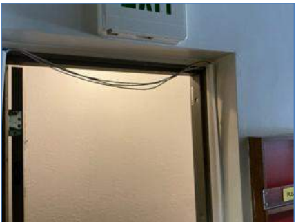
Exhibit 15 - Exposed cables above doorway.
