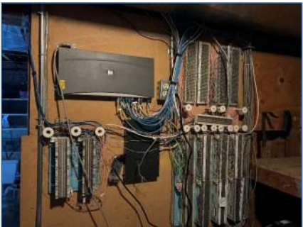
Exhibit 13 – Lower-level telecom equipment
