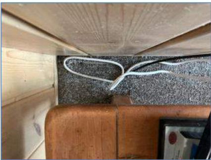
Exhibit 15 – Coax cable punched through floor
