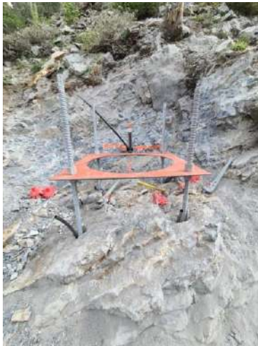
Wyssen footing disturbance
