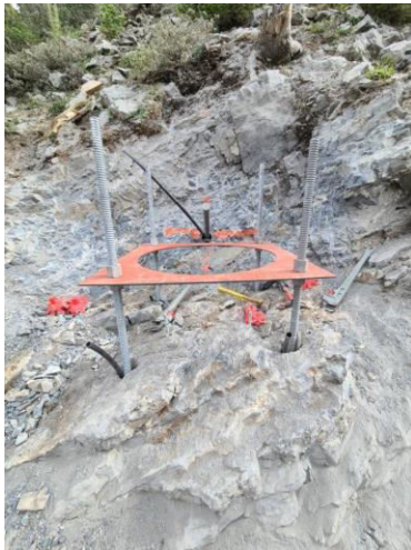
Wyssen footing disturbance
