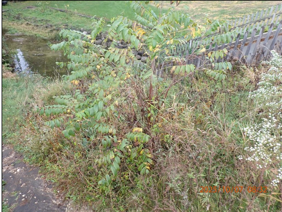
Waterville Dam Woody Vegetation On Left Downstream Embankment 0022110072515.JPG
