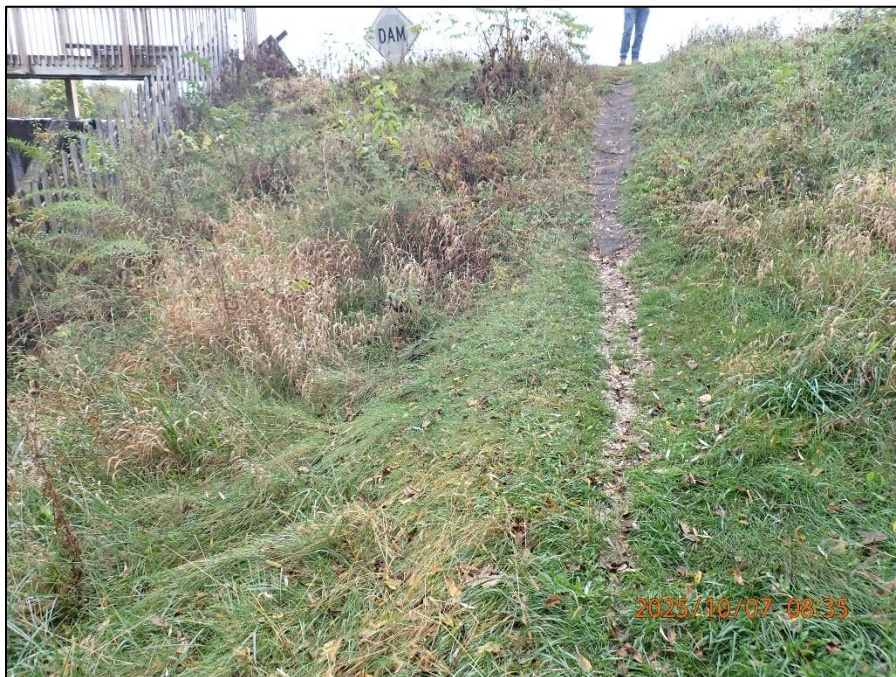
Waterville Dam Rutting from Pedestrian Traffic On Left Downstream Embankment 0022110072514.JPG
