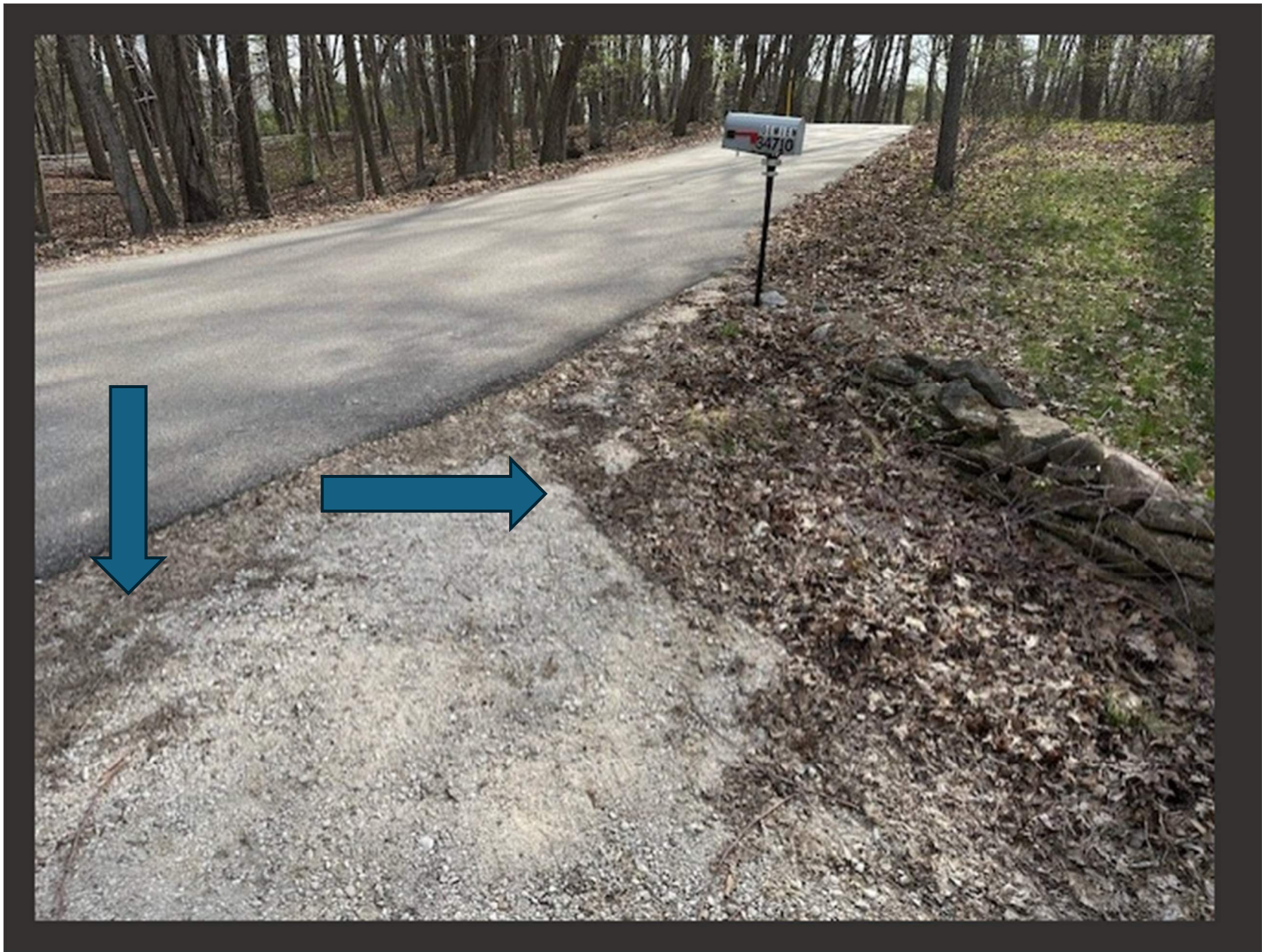
TAPER OF OLD GRAVEL DRIVE UP TO ROAD WITH ROAD IMPROVEMENT CAUSED EROSION.
