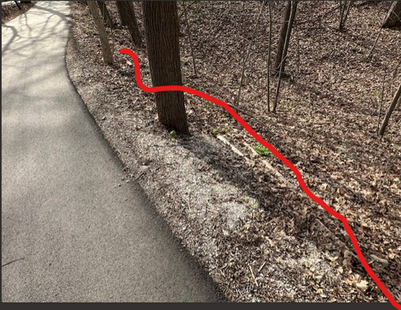
FURTHER ROAD BASE WASH OUT
