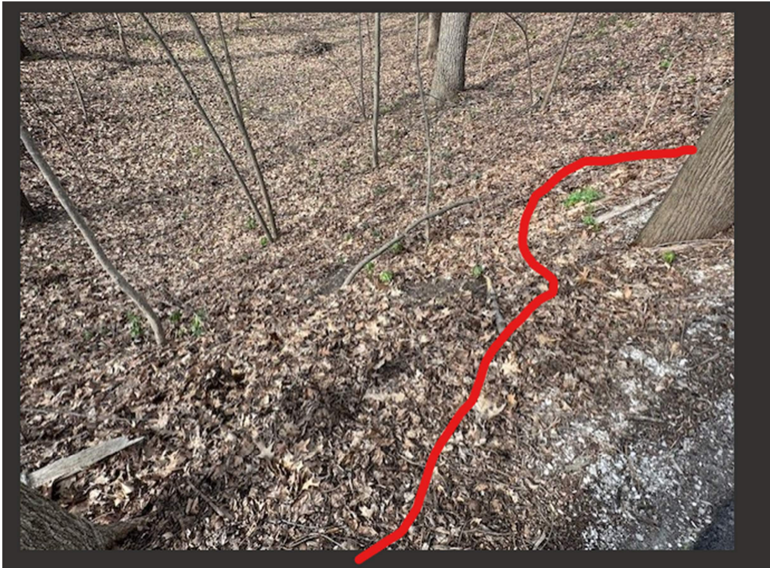
ROADWAY GRAVEL WASH OUT 1 MONTH AFTER ROAD PLACEMENT
