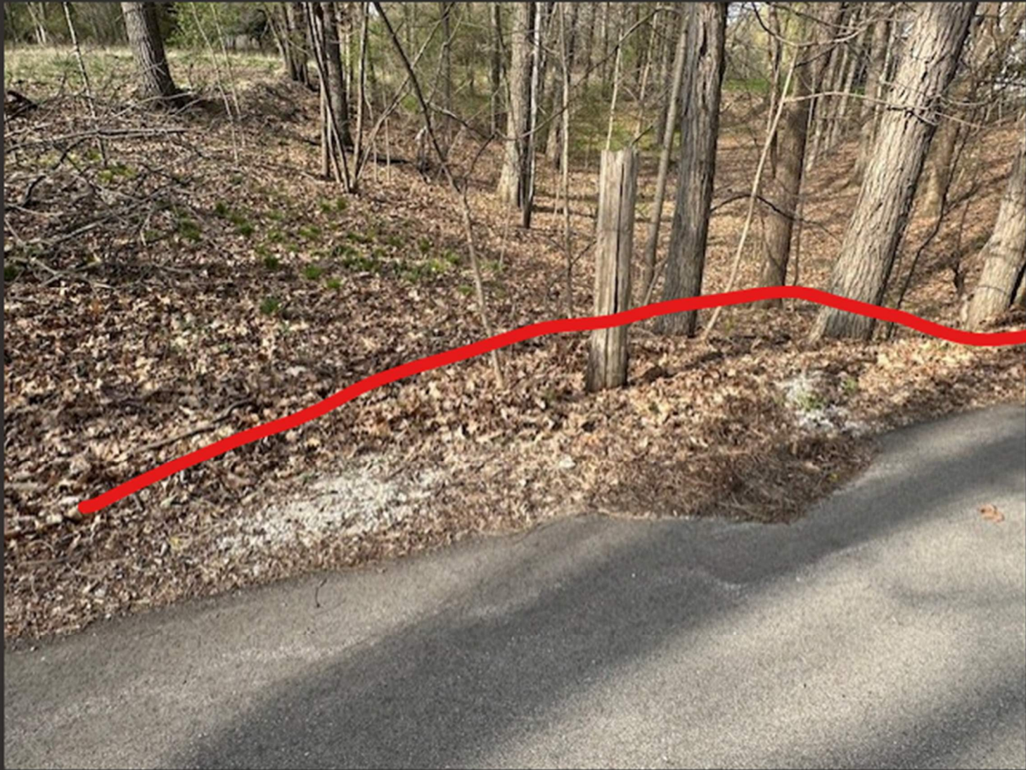
ROAD BASE HAS ERODED INTO THE 34710 LOT AND NO LONGER MAINTAINS THE 12" SIDE GRAVEL, BUT HAS EXPANDED TO 18-24" IN WIDTH ONTO THE PROPERTY NORTH OF BARTLETT ROAD.
