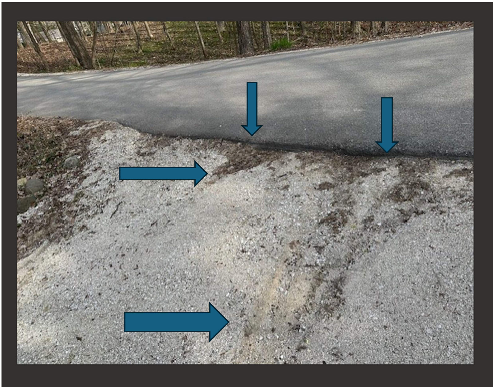
DRIVEWAY WASHOUT AFTER THE ROAD REPAVEMENT, BUT BEFORE THE MAJOR 2025 STORMS. AFTER THE STORMS THESE DROPS OFF PAVEMENT WERE 4-6" IN DEPTH.
