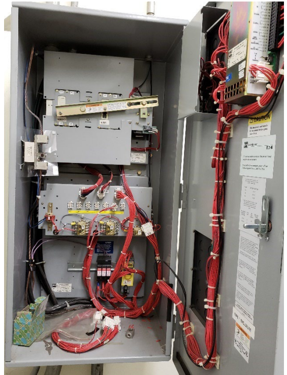
Photo 2 Inside the existing ATS panel.
