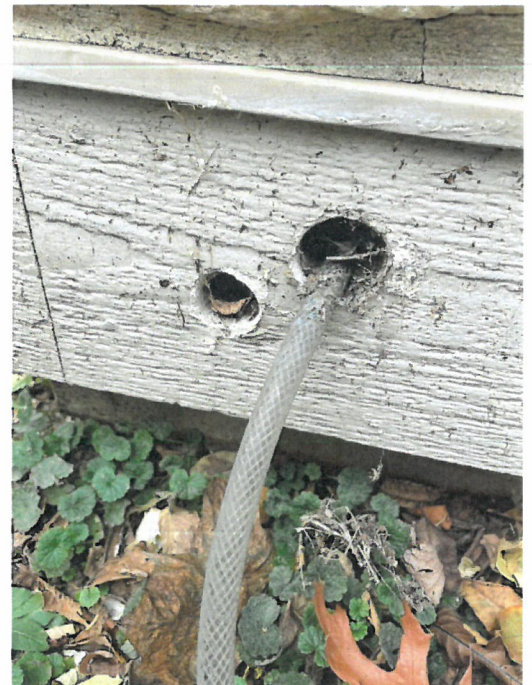
Photo 4 Lift Station No. 5: Exterior holes
