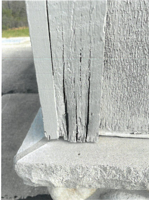
Photo 5 Lift Station No. 6: Siding batten strips dried out and deteriorated.
