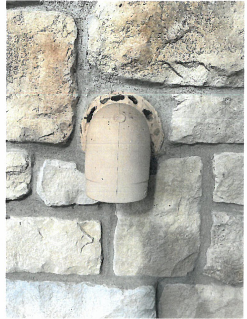
Photo 2 Lift Station No. 2: Existing sealant pulling away from exterior vent.
