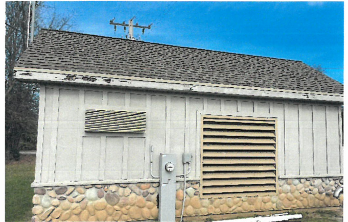
Photo 6 Lift Station No. 6: Southside wood fascia damaged.
