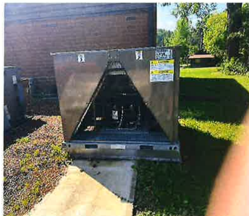
TAGS: HVAC; COMMENTS: New Condensing unit not properly set on existing pad
