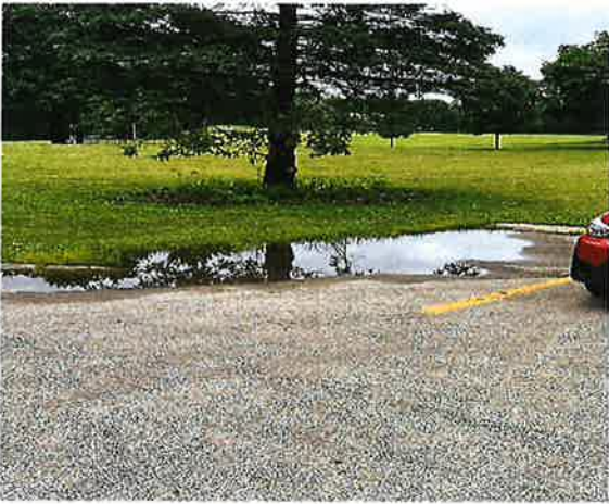
TAGS: Landscaping COMMENTS: Ponding issue after rainstorm NW upper parking lot
