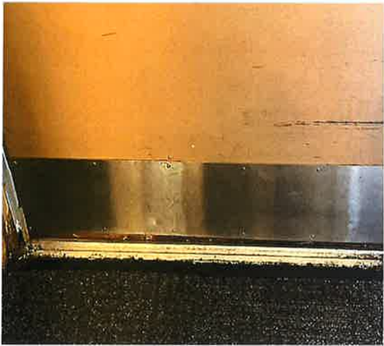
TAGS: Interior COMMENTS: Staff entryway door in need of replacement
