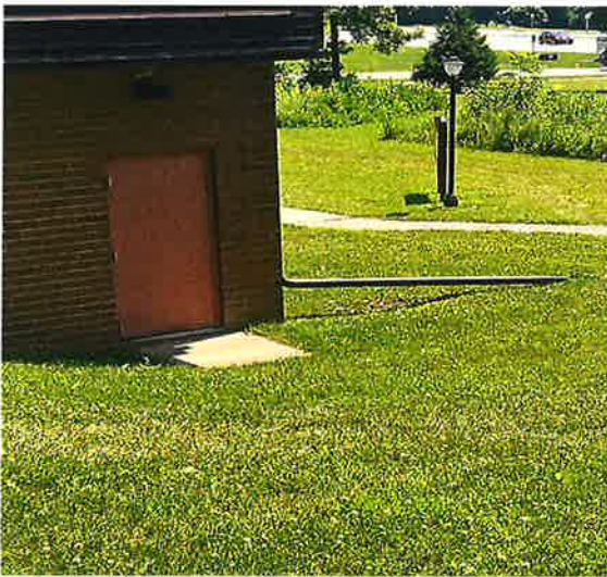
TAGS: Landscaping COMMENTS: SW corner lower level. Pitch causes water to pond near building. Gutter terminates in upslope
