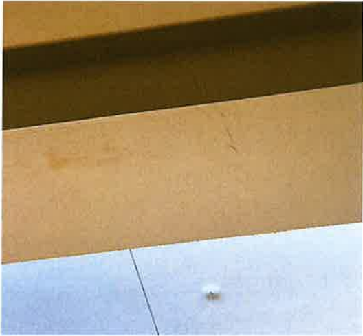
TAGS: Interior COMMENTS: Drywall damage at ceiling typical several
