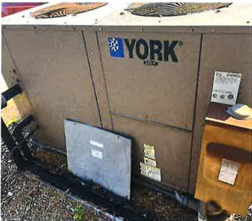
TAGS: HVAC COMMENTS: Electrical Cabinet panel cover not put back in place//
