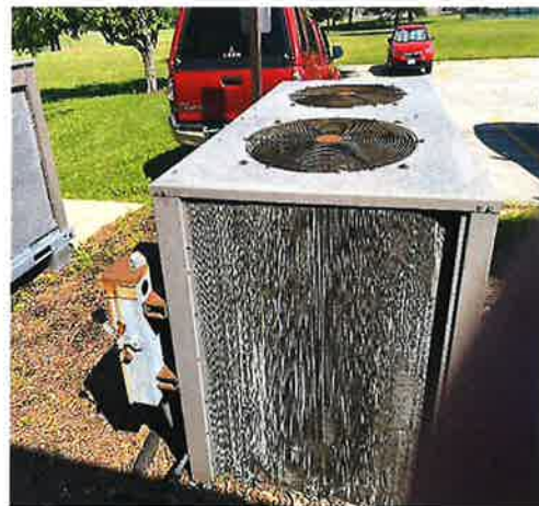
TAGS: HVAC COMMENTS: Fin and coil damage
