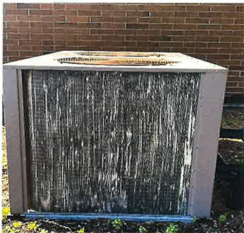
TAGS: HVAC; COMMENTS: AC-1 Lower Level. Coil damage from chemical and power washing
