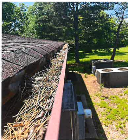
TAGS: Landscaping COMMENTS: Gutter condition typical North Face gutters
