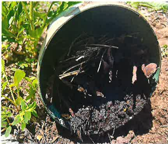
TAGS: Landscaping COMMENTS: Collector outlet from NE downspouts
