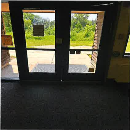
TAGS: Interior COMMENTS: Lowerlevel entry door does not seal. Will not open properly.
