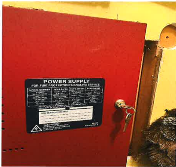
TAGS: Interior COMMENTS: Wall penetration needs to be sealed properly.
