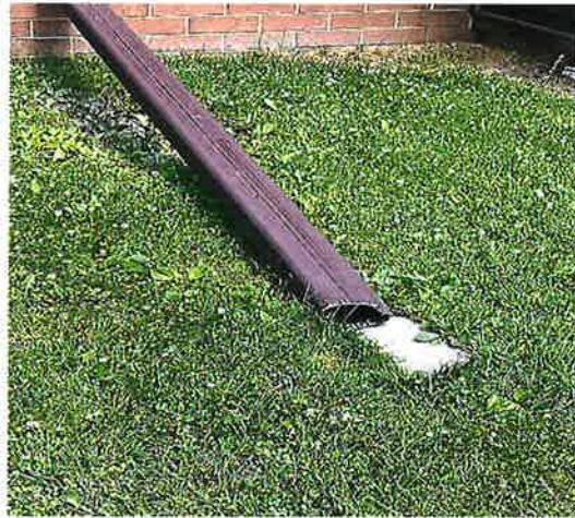
TAGS: Landscaping COMMENTS: Gutter terminated on upslope. Pitch traps water at building.
