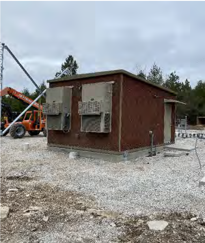
Fish Creek Tower 12x20 Shelter
