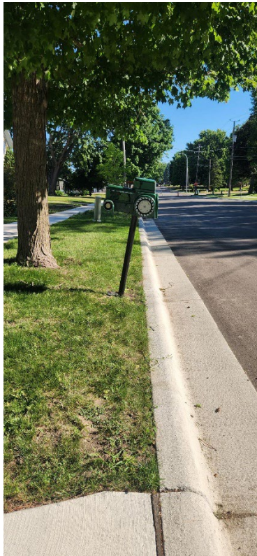
Mailbox improperly installed, weed control and seeding inadequate
