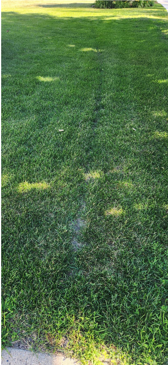
Photo illustrates poor restoration
