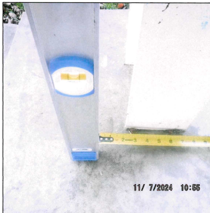
Figure 4. Columns roughly 2 in. out of plumb.
