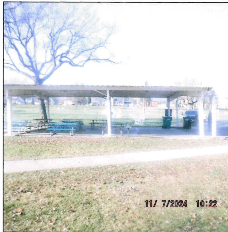
Figure 4. Shelter visibly leaning to the south (left).
