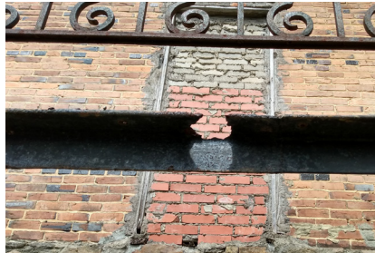
Spots around the supporting framework have entirely rotted away.
