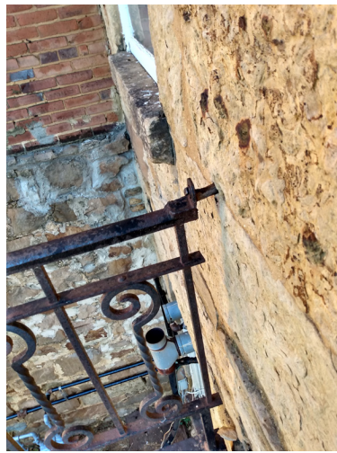
West railing top has an insecure bolt that has moved ~1.3 inches away from the wall.
