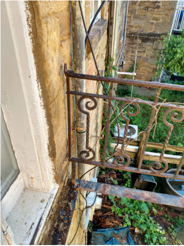
East railing top is detached from the wall.
