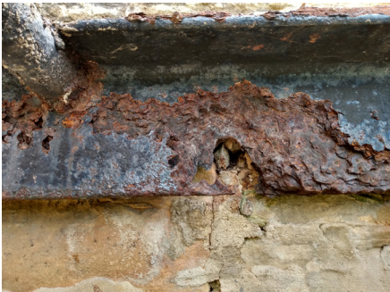
A severely rotted bolt slid out of place from the center hole (of 3) in the (also rotted) angle iron ledger when we tried to turn the nut.
