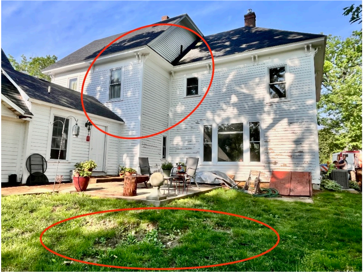
Grounds deterioration from water run-off
