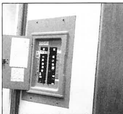
Figure 2 – Front Office Load Center
