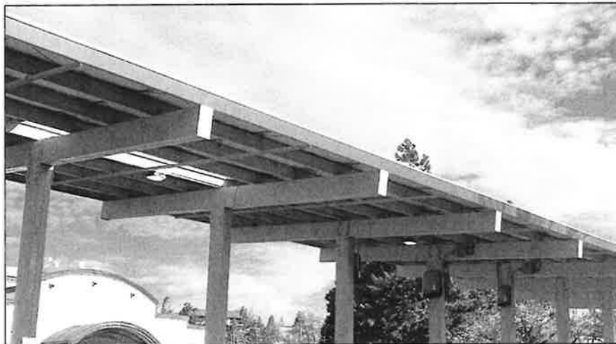
Figure 5 – Existing PV Array
