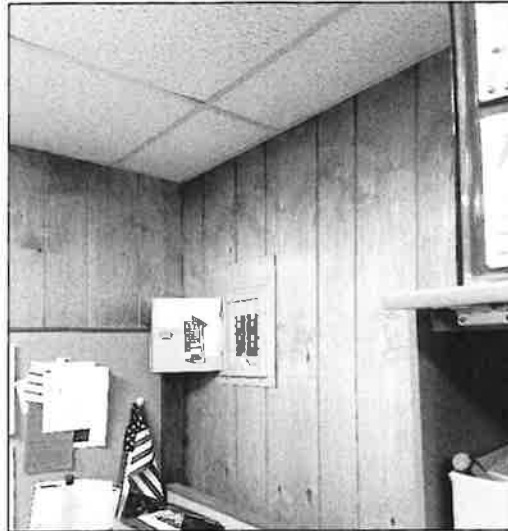
Figure 3 – Inadequate Panel Placement
