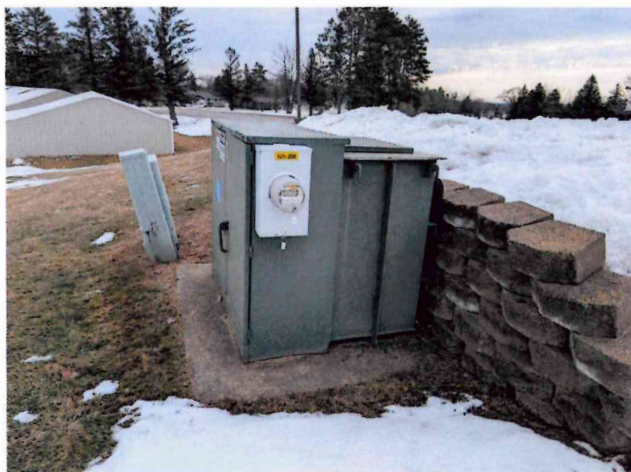
Photo of transformer and meter
