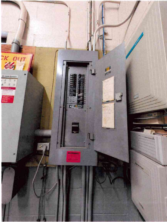
Photo of main service panel
