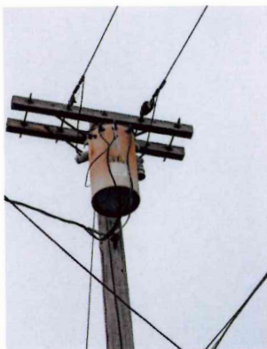
Photo of transformer
