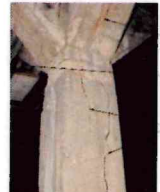
P1 DAMAGED COLUMN SCALE
