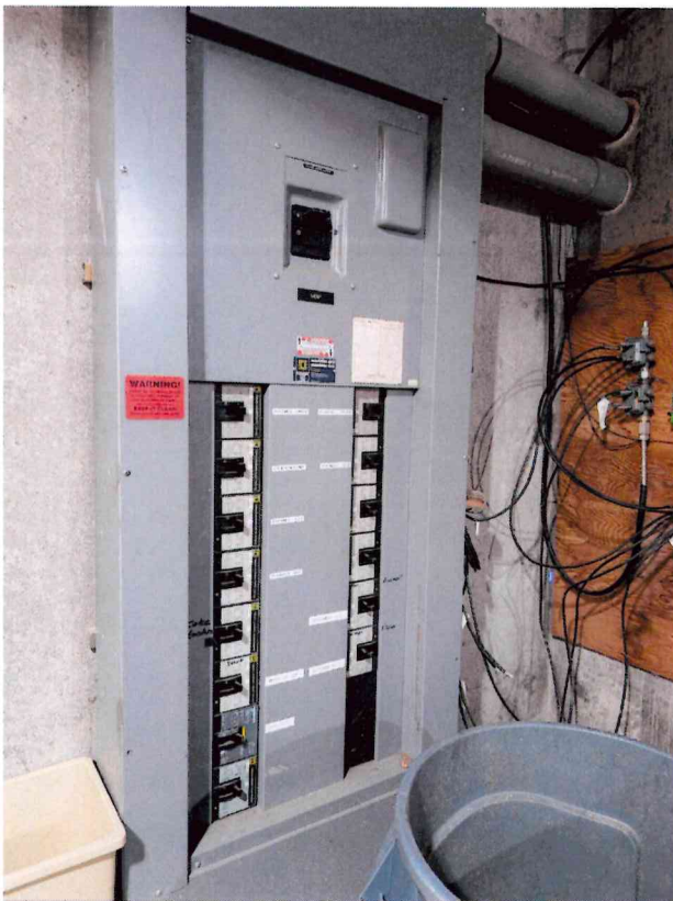
Photo of main service panel
