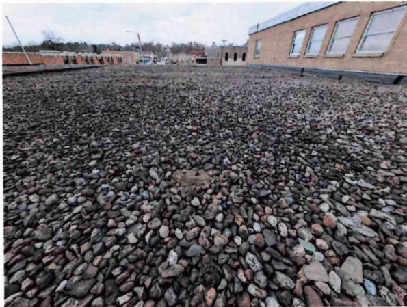
Photo of unadhered river rock
