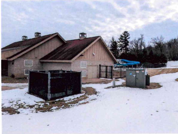
Photo of meter and transformer
