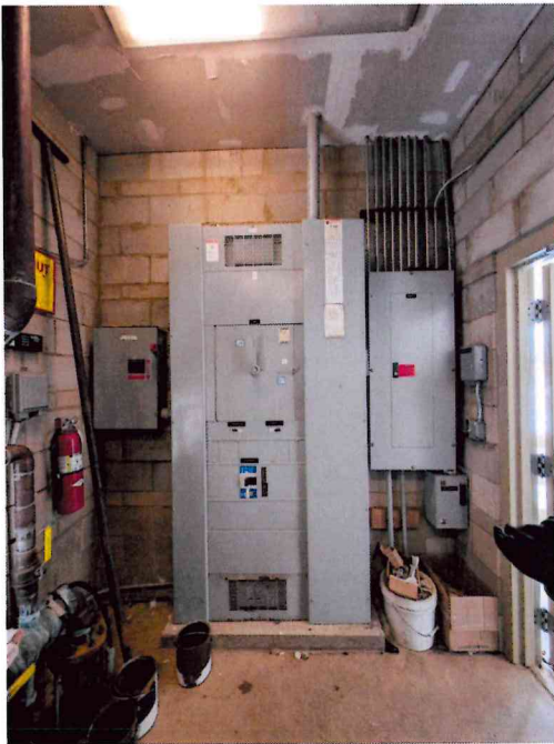
Photo of main service panel
