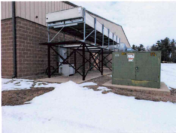
Photo of meter and transformer
