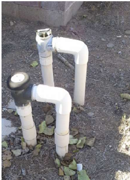
Wrong or Missing Backflow Preventer on Irrigation
