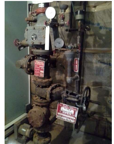
Missing/Wrong Backflow Preventer on Fire System
