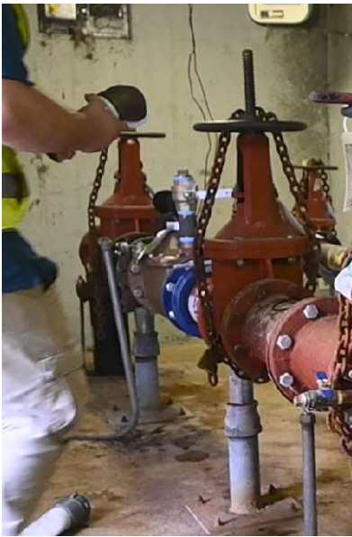
Missing Backflow Preventer at Meter
