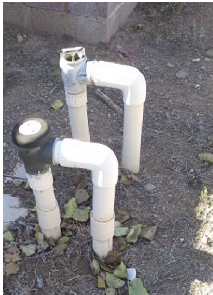
Wrong or Missing Backflow Preventer on Irrigation
