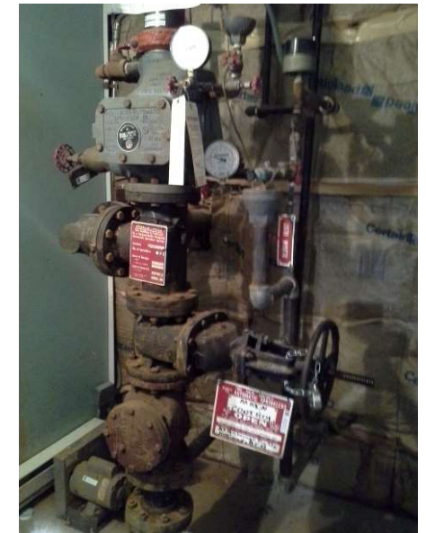
Missing/Wrong Backflow Preventer on Fire System
