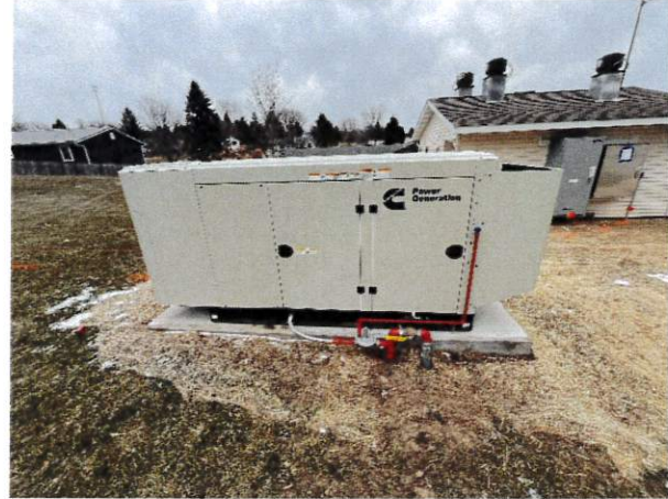
Wellhouse #2 Generator: February 24, 2026
