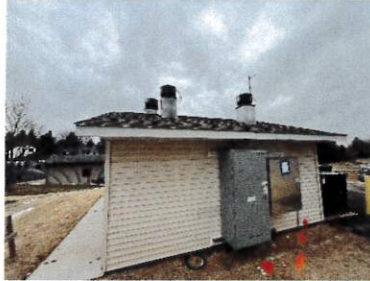
Well #2 Electrical Service Gear
