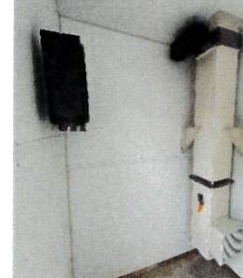
Well #2 Chemical Room (New)
