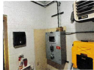
Well 1 (Tower) SCADA Panel
