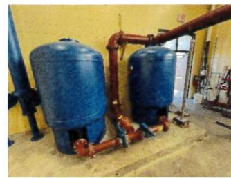
Booster Station Pressure Tanks
