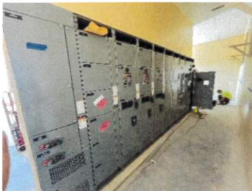
Wellhouse #3 Motor Control Equipment
