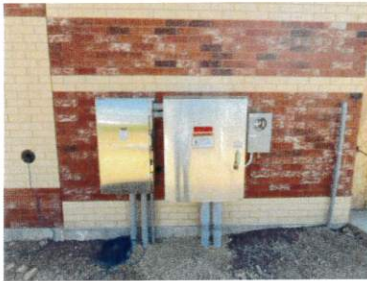
Electrical Service Gear
