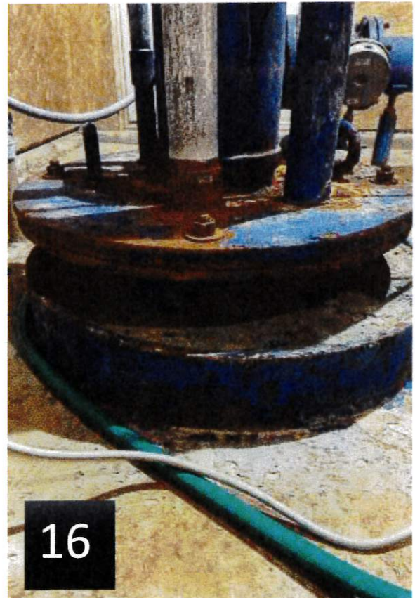
Concrete collar surrounding the casing appears less than 6" and casing terminates less than 12" above floor and deeper than 10' into ground per well construction report
