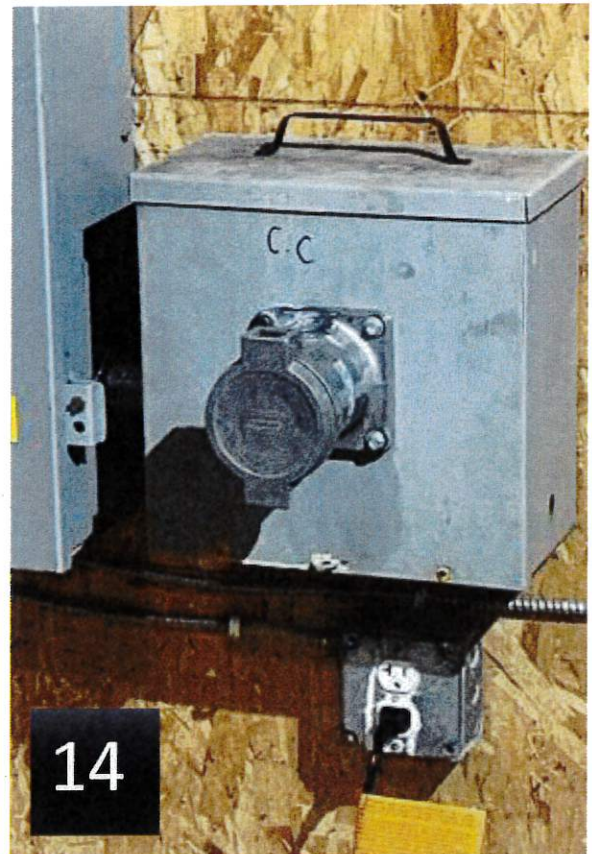
Emergency power for well 2 inside well house
