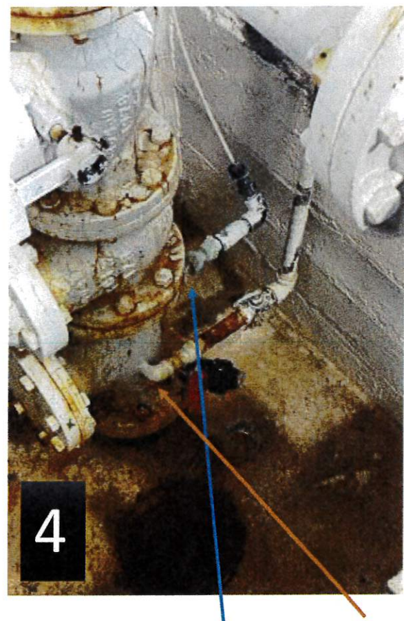
Chemical injection location and EP tap plumbing (nonconforming)
