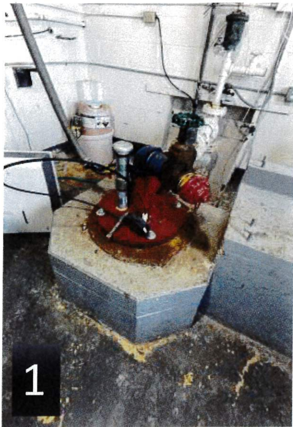
Well 1 with 2" vent
