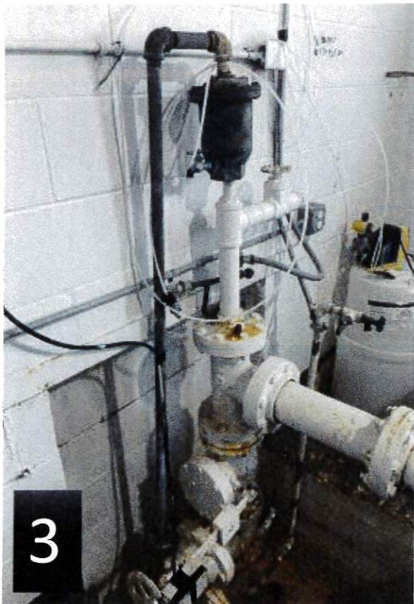
Air vacuum relief valve with raw tap. Request discharge pipe be raised to be >24" from main well house floor.
