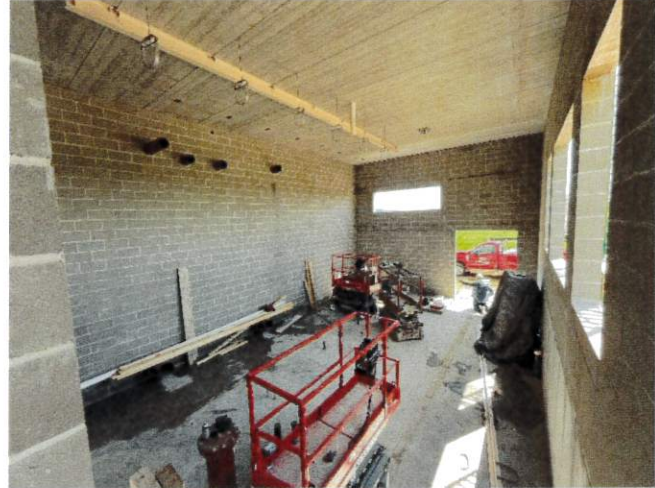
Wellhouse #3: Booster Room, July 2025
