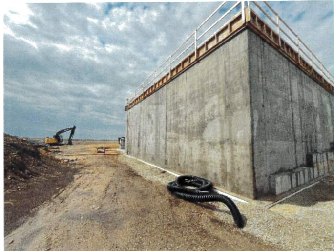
WELLHOUSE #3 FACILITY: April 2025
