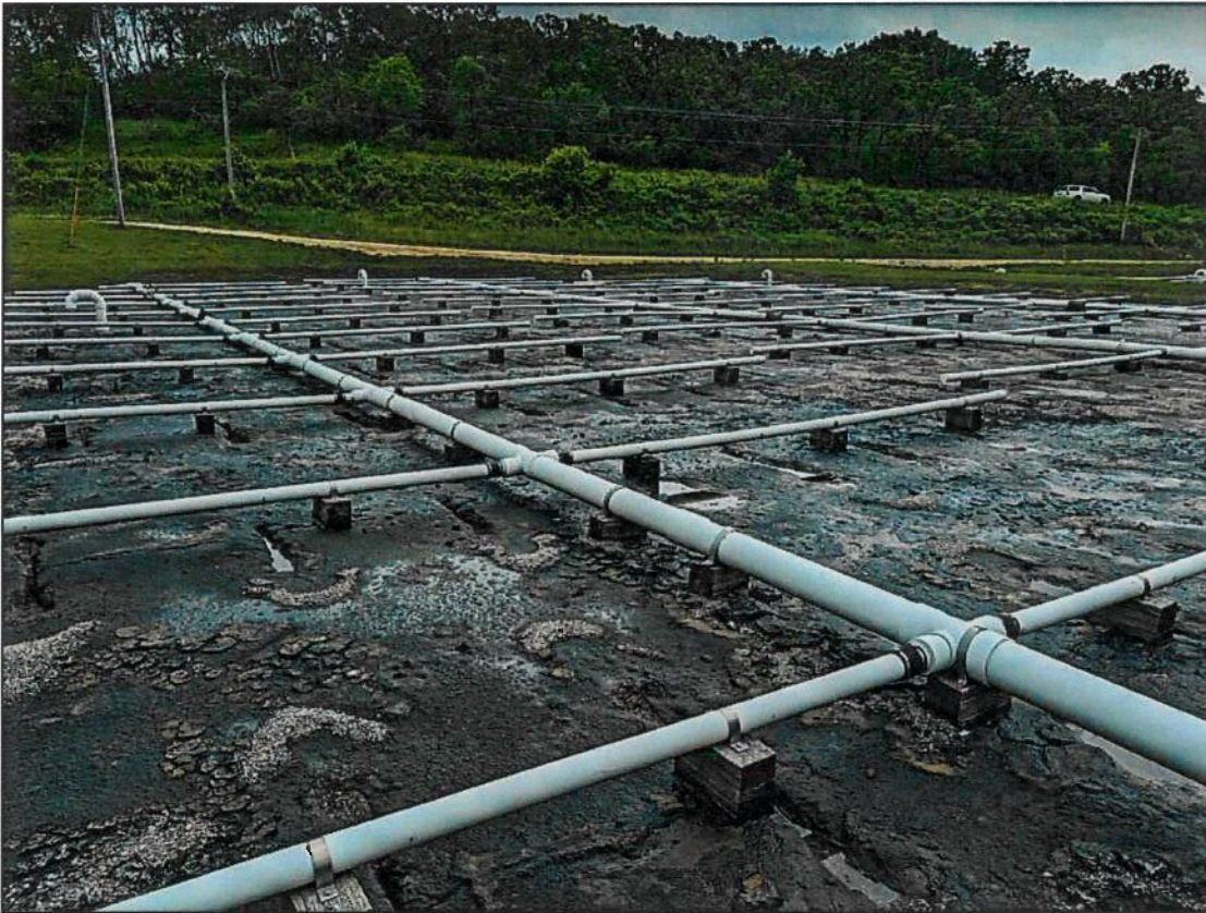
Figure 4. RSF media in 2024 (showing sludge discharged to RSF)
