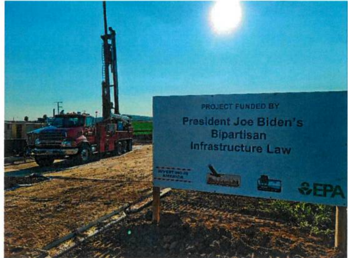
SDWLP FUNDING SIGN AT WELLHOUSE #3 SITE
