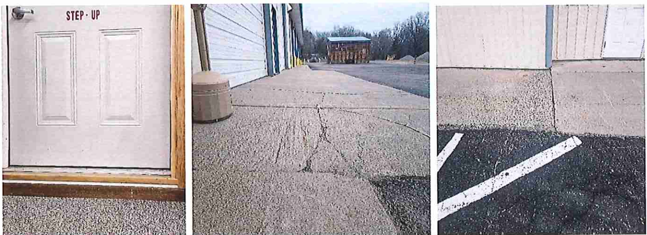
CITY HALL & BREEZEWAY ELEVATION ADA ACCESS ISSUES.
