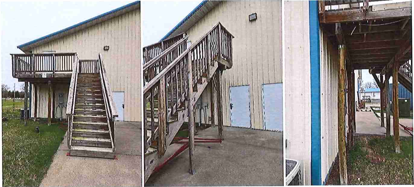
FIRE STATION REAR COMBUSTIBLE DECK.
