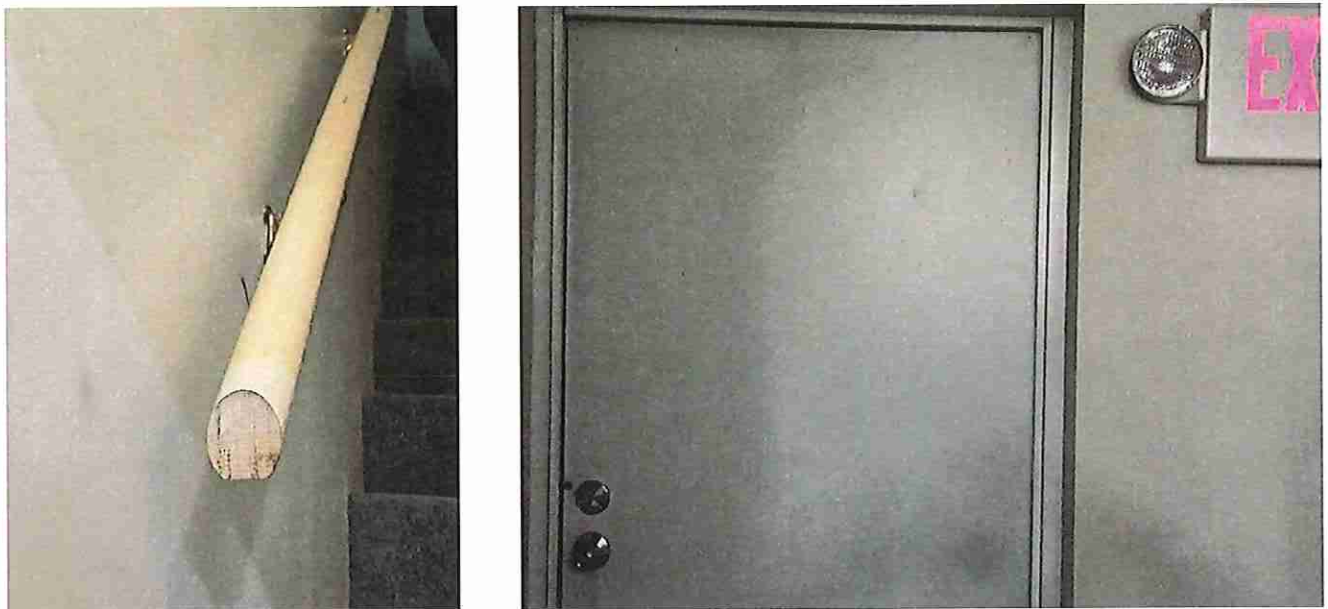
FIRE STATION NON-COMPLIANT HANDRAIL, REAR EXIT DOOR, & DOOR STOPS.
