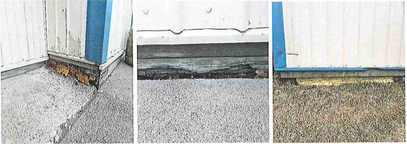
PUBLIC WORKS & CITY HALL UNPROTECTED FOUNDATION AND DETERIORATION.
