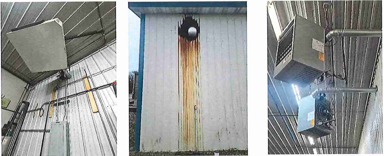
PUBLIC WORKS HANGING HEATERS WITHOUT DRIP CAPS & LEAKING.
