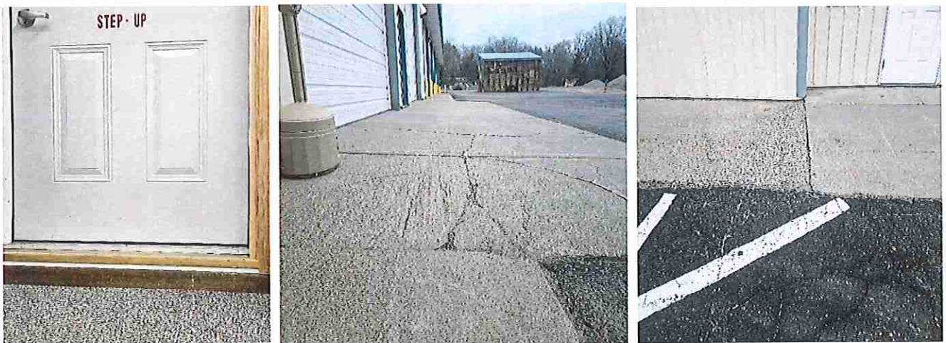
CITY HALL & BREEZEWAY ELEVATION ADA ACCESS ISSUES.
