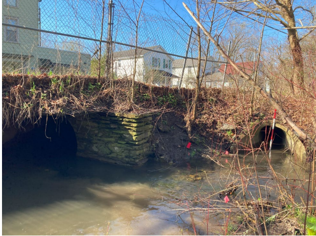
Photo 27: ETWBDSCF on 4/15/24. Downstream View. ETWBOT1 visible. Stadia rod for scale. Rte. 343 above downstream crossing structure.
